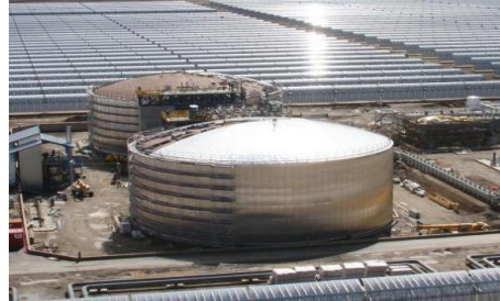
Dual tank molten salt storage of Andasol I
